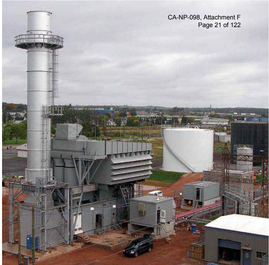
Maritime Electric's new 50-MW combustion turbine generator will provide increased reliability and security of energy supply on Prince Edward Island.
